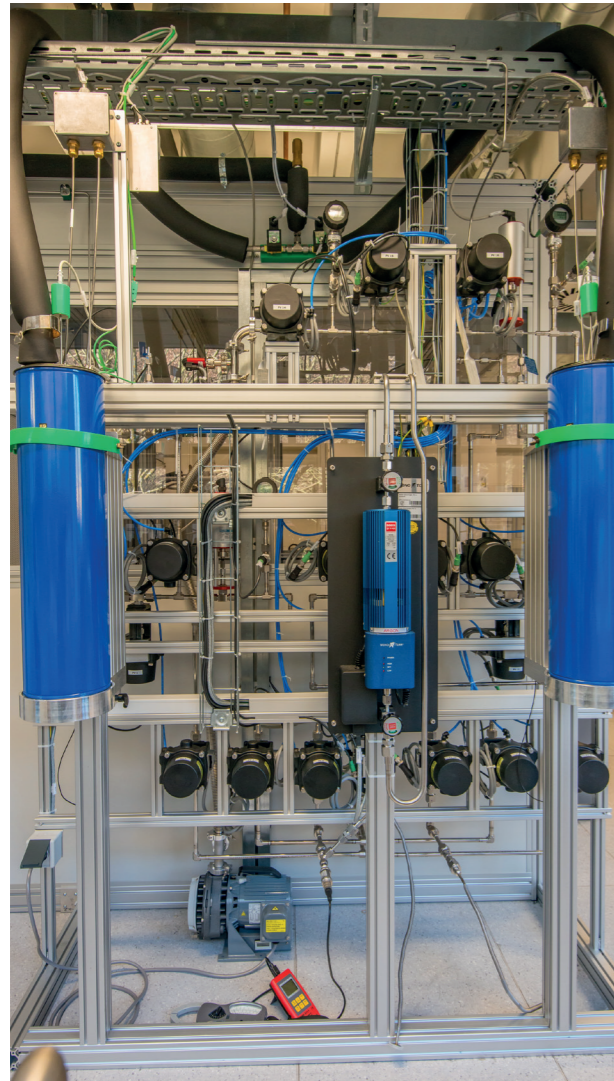
Fig. 6: The new automated emanation system (Auto-Ema). The piping and instrumentation is in front of the clean box containing the sample vessels.
