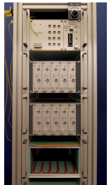
Fig 8: Rack setup featuring ten STAREP channels with controller and reference.
