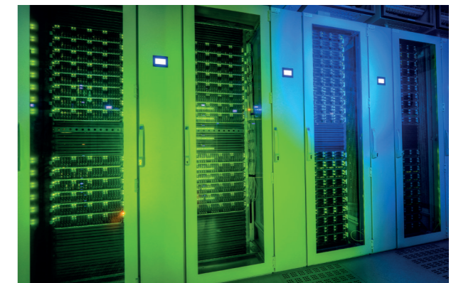
Fig. 1: Four water-cooled racks containing the 272 servers of the two clusters. The new cluster is located in the two leftmost racks.
